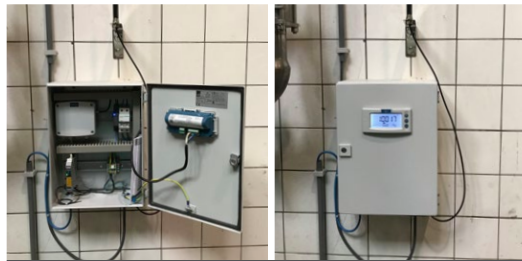
M853 DAC-Module and D077 Level Monitor
