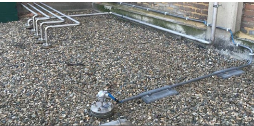
Level Sensor in hazardous area
