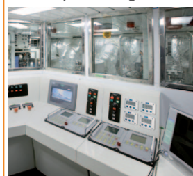
Flow Computers in engine room
