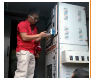
Generator instrumentation panel
