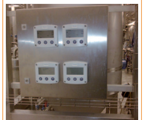
Fluidwell solution on location
