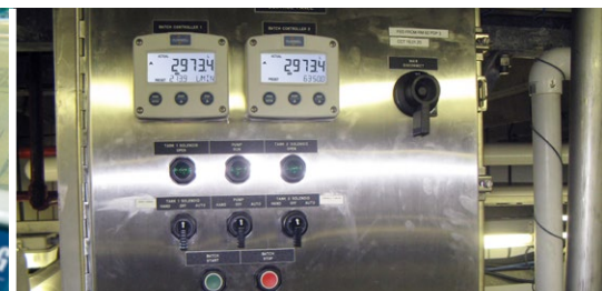
Remote controlling from process control panel.
