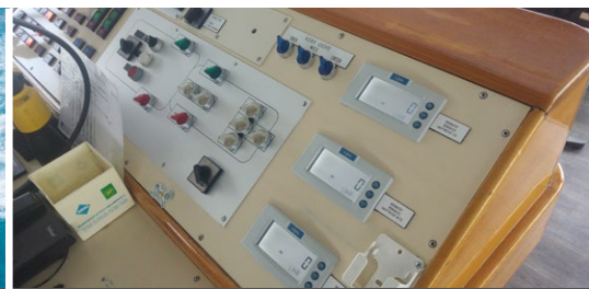
Display real-time fuel consumption on the bridge
